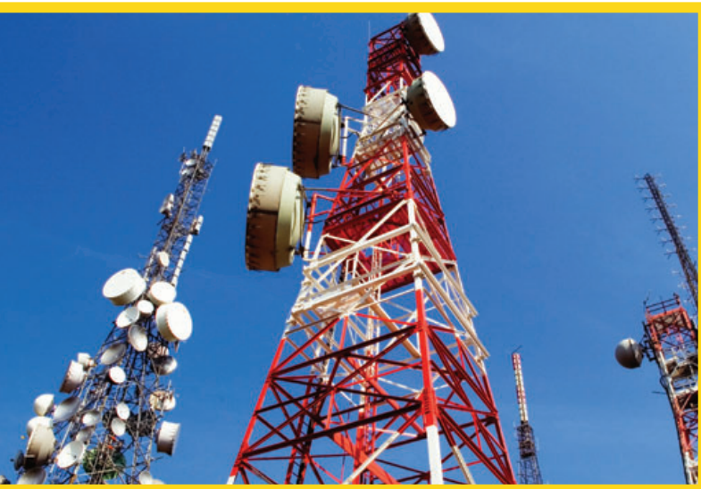
⤴ A cell tower
